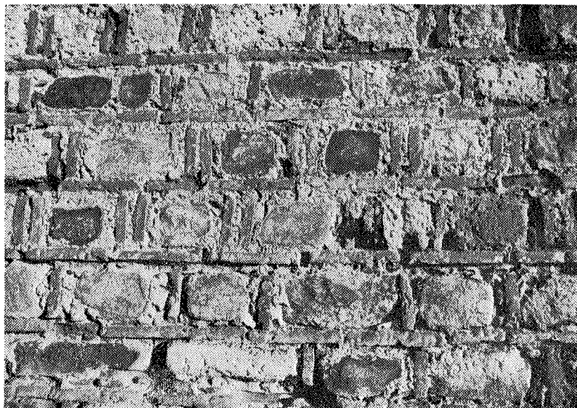
5 Ilca - Loutra, Khan of Ghazi Evrenos Bey, late 14th century, detail of the masonry.
